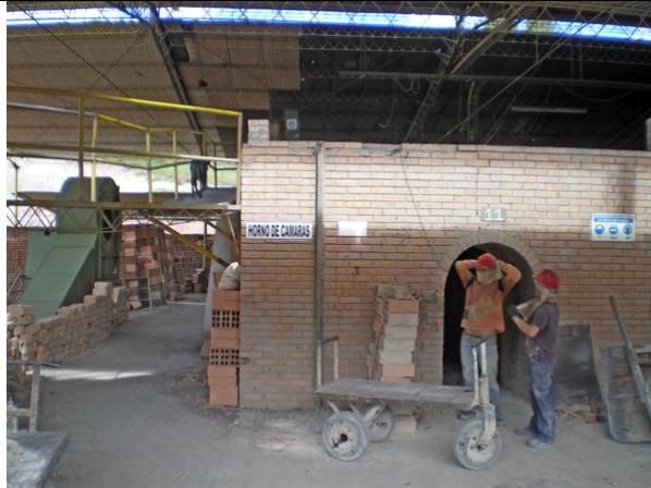
Figure 4. Chamber kiln at Santander Ceramic (project situation).
